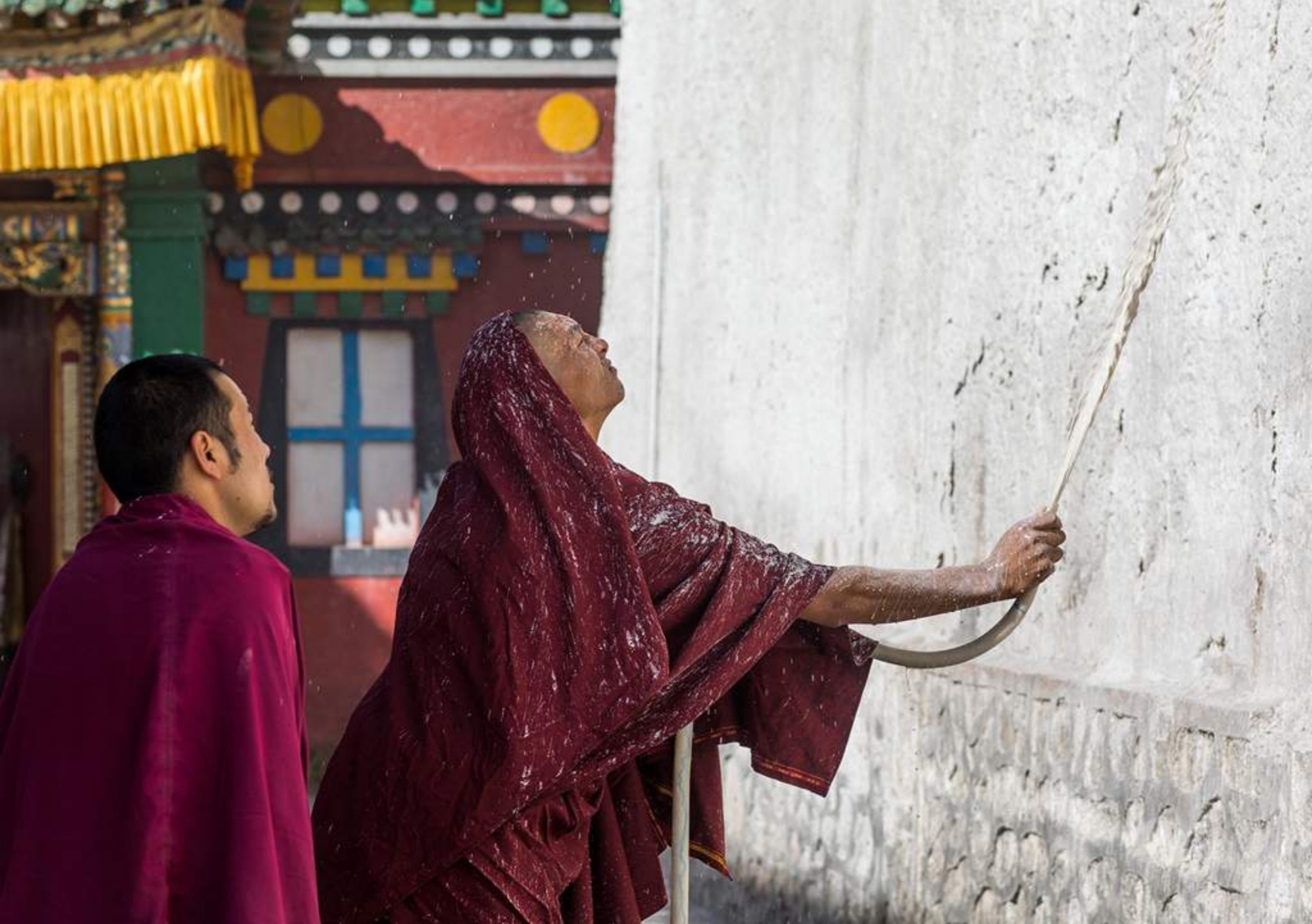
Then, the monks spray the mix onto the temple walls to make it look white and new.
