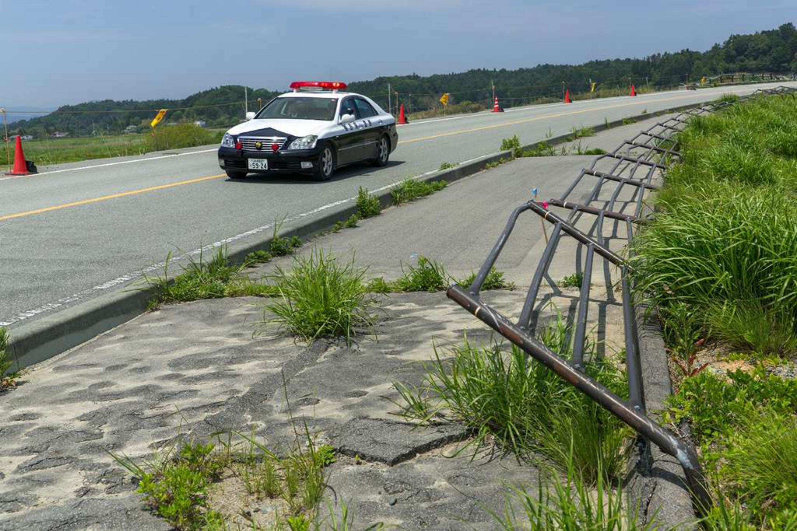
Road barriers were bent out of shape by the powerful waves. Only the police still patrols in the area to monitor the few houses that are still standing and to control curious visitors. In the distance, speakers encourage workers to consult a doctor in case of persistent migraines.
