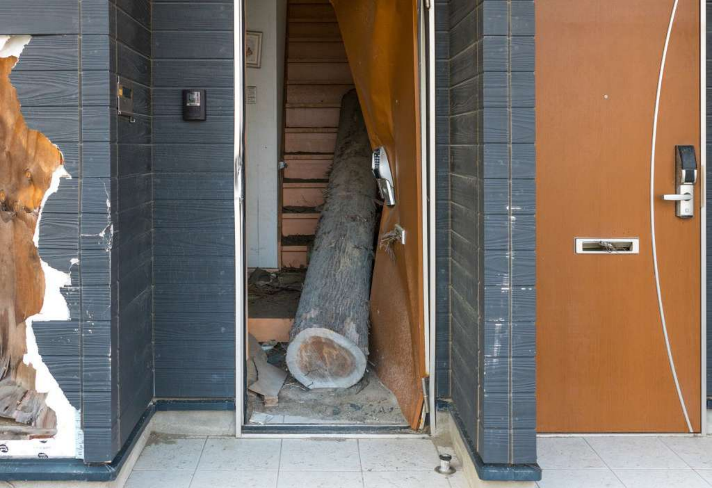
Five years later, the scars of the tsunami are still visible, like in the town of Tomioka. The law now prohibits living in areas destroyed by the tsunami. Only industrial or commercial activities are allowed, but very few have applied.
