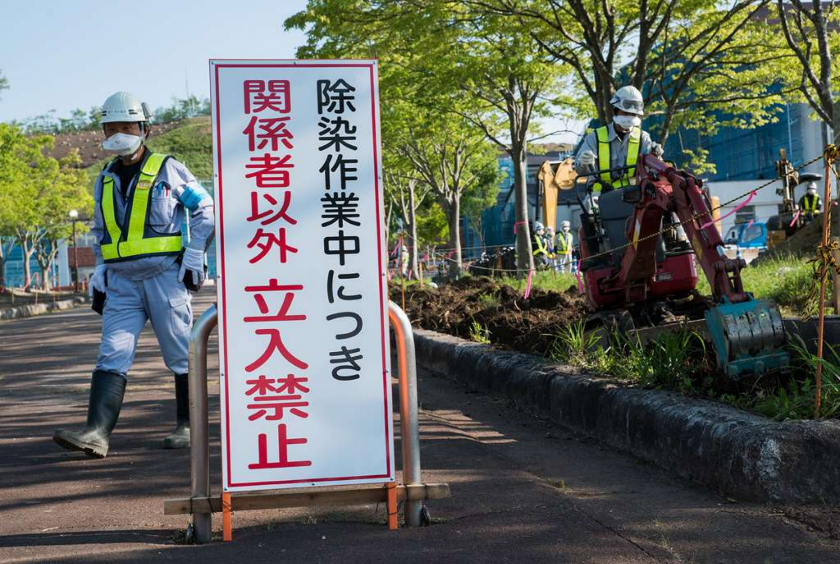
Workers are decontaminating a school in the town of Litate: « we remove 5 to 30 cm of soil and put it in plastic bags, which we store on the outskirts of town, pending a better solution. ». A full year of work will be necessary to make the school clean again. Only workers have been living in Litate for now...
