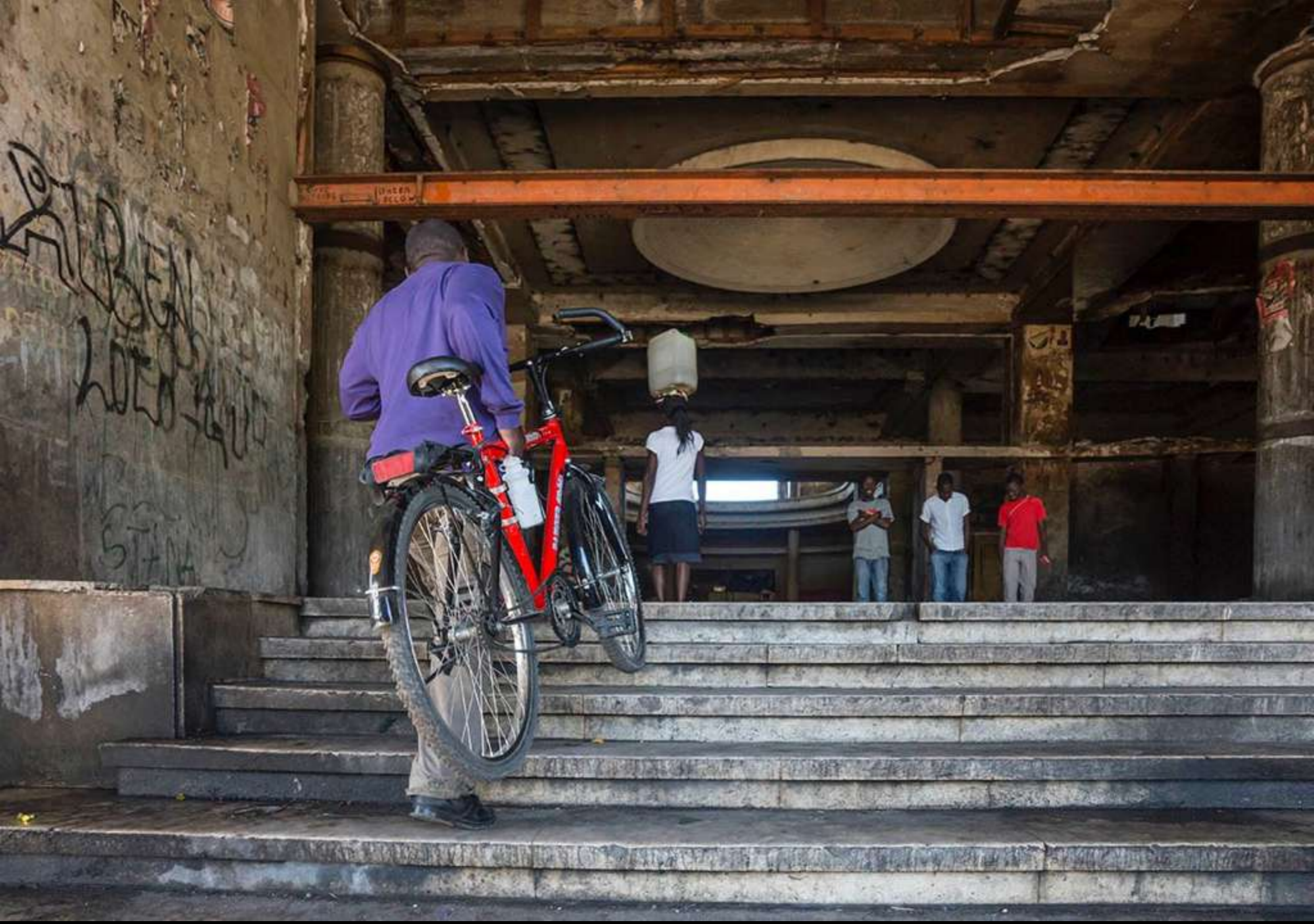
The living conditions are atrocious. Drugs, disease, and trash are ubiquitous. People have removed much of the plumbing, electrical, windows and even concrete to sell on the black market. This weakens the building but provides them with another meal.
