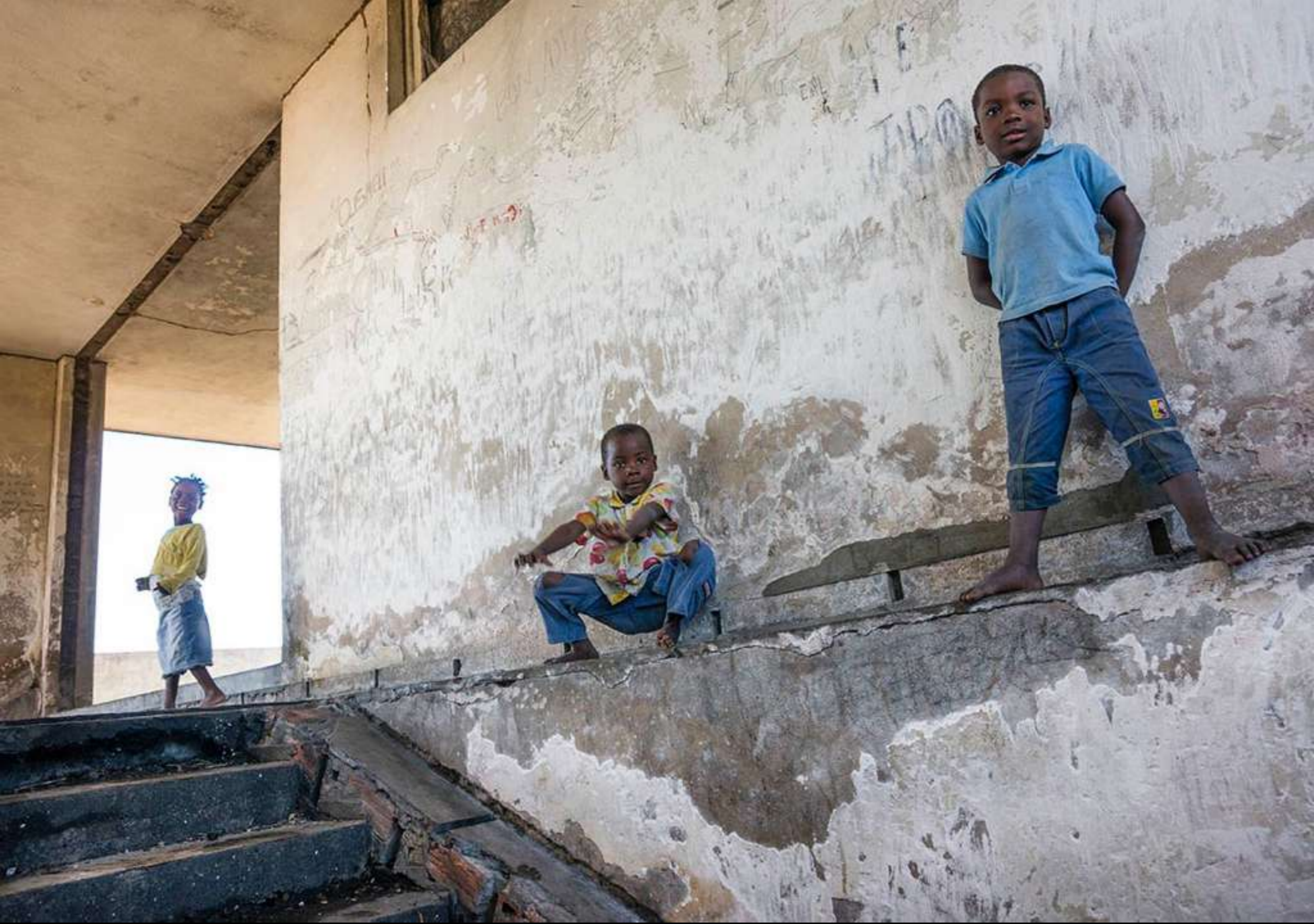
Children play around open elevator shafts with... no elevator in sight! "No one knows when the building is going to collapse," says one resident, "It's going to collapse on top of our poverty".
